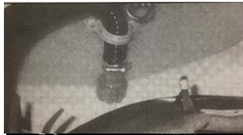
Figure 8. Finished installation of the strum box against the bulkhead at the back of the cockpit.
