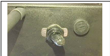
On/Off switch and fuse on side of electrical junction box. Figure 2
