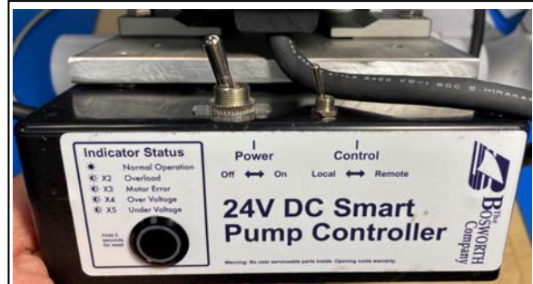
Pump Control box showing manual and remote activation switches on top of box and fault status indicator on side Figure 6
